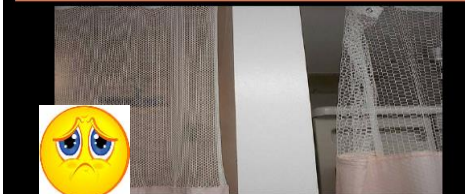
Sprinkler- Curtain Mesh
